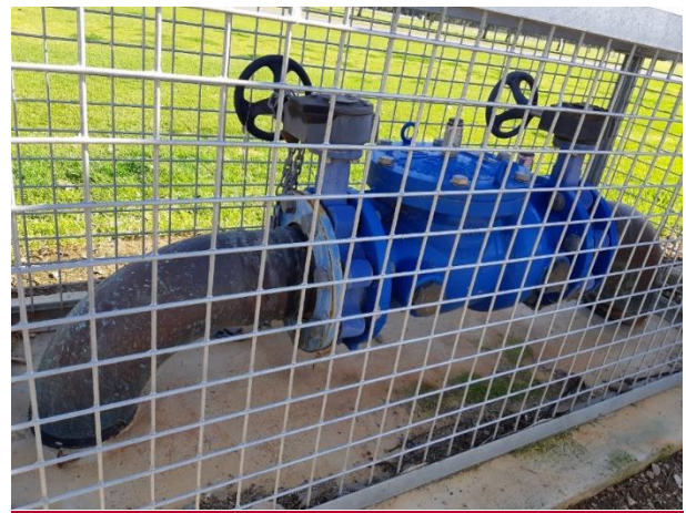
Figure 5: Glenelg-Adelaide Pipeline Valve.
