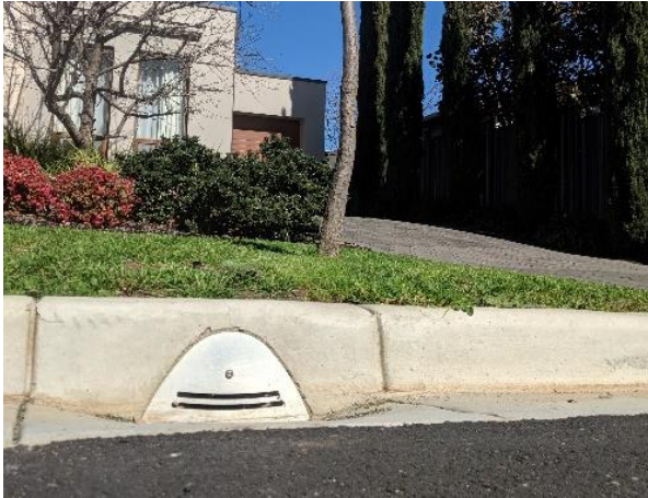
Figure 7: Kerbside infiltration – tree inlet, Glenunga, City of Burnside
