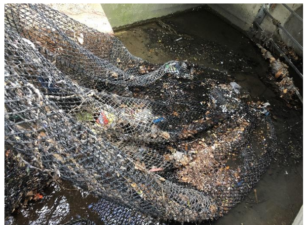
Figure 12: Gross Pollutant Trap (GPT), near Morphett St Bridge, City of Adelaide.
