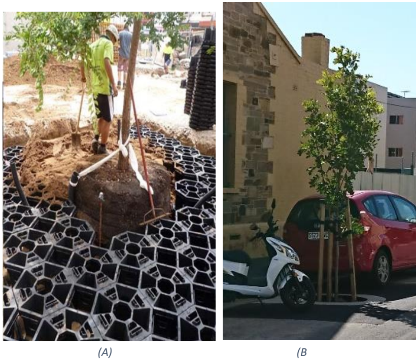
Figure 5: Examples of how the councils create more space underground for trees in contested environments to help support the growth of a tree. (A) Cutting into the road space to put a tree strata cells that support stabilization of the soil when - (B) bitumen goes on the top, and therefore leaving space for car parking either side of the tree;
