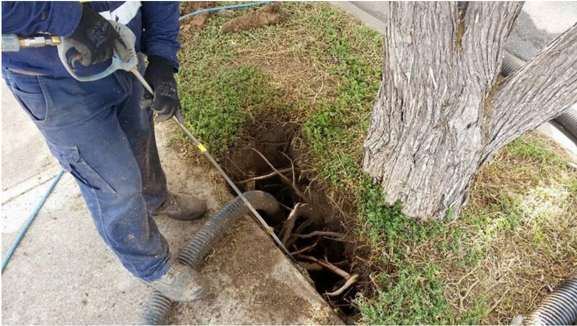
Figure 17: Vacuum excavation used to expose tree roots next to a footpath. Image: https://southvac.com.au/hydro-excavation/
