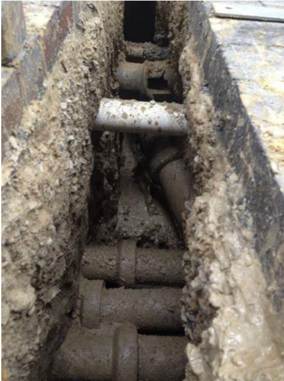
Figure 12: Example 1 of the extent of services in a city underground space, Bank Street Adelaide.
