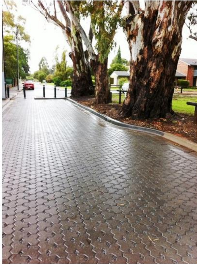
Figure 8: Example of permeable paving above underdrains that direct storm water into the adjacent reserve and into the road subgrade. The construction is laid close to mature trees with no damage to paving surface. Image taken from Lawry et al. (2017, p.6)
