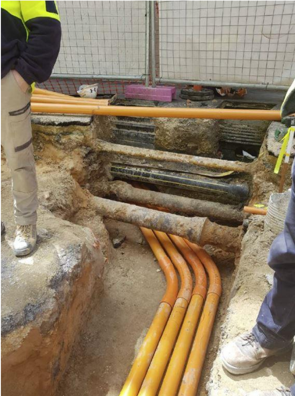
Figure13: Example 2 of the extent of services in a city underground space, Bank Street Adelaide.
